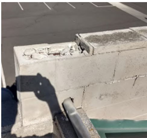
Missing masonry cap, weather damaged mortar
