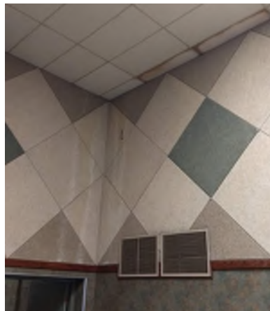
Water staining from roof leaks
