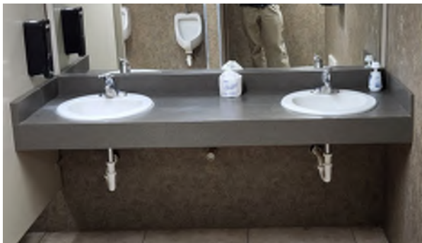
Wear and staining on Men's vanity top
