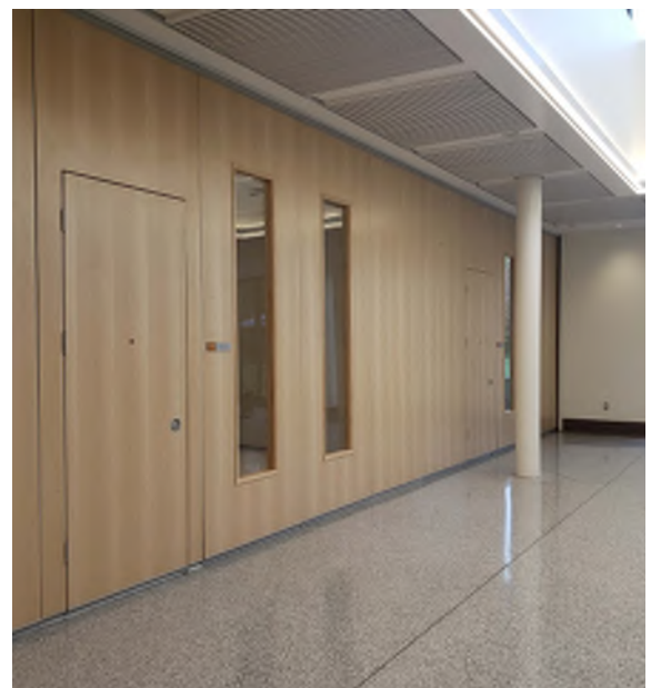
Picture of folding partition with egress door in one of the panels
