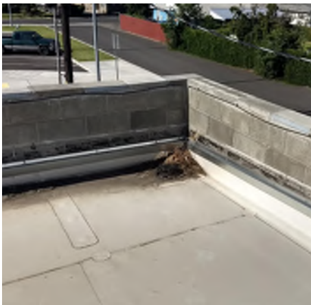
Lower roof drains should be cleaned
