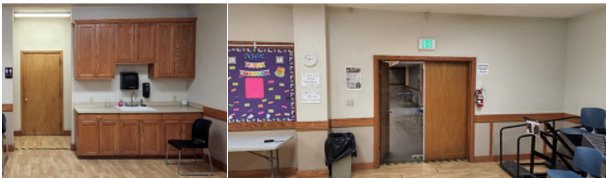
Pictures of warped floor and gaps
