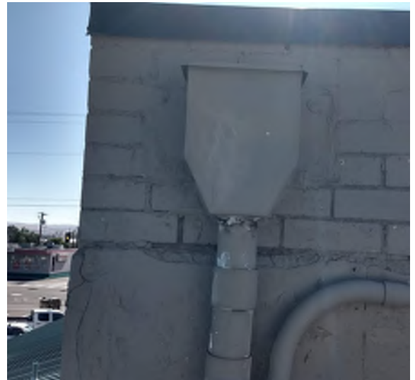
Collector head and piping
