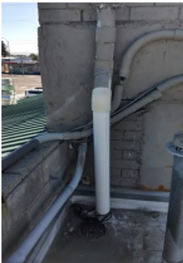
Damaged masonry and grout at drain piping
