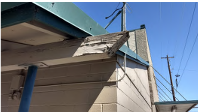
Weather damaged exposed beam and vertical wood siding
