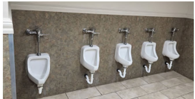
Urinals, recommend adding privacy screens
