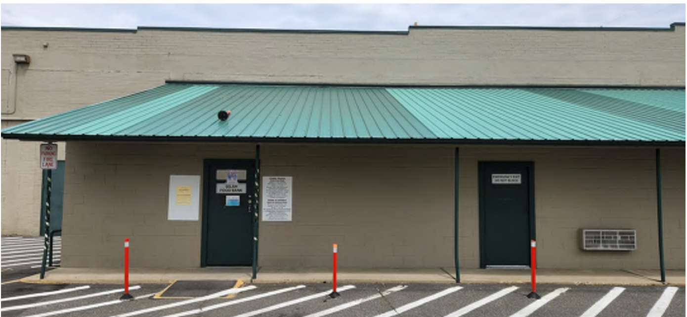
Mismatched metal roofing panels, and stepped parapet of the main or high roof
