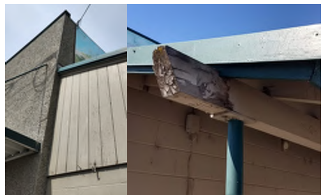
Weather damaged exposed beam and vertical wood siding
