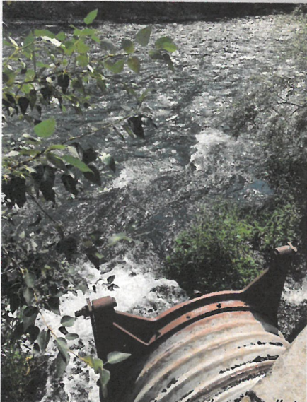
Storm drainage pipes often discharge pollutants, such as bacteria, fertilizers, and everyday household chemicals into local waterways.
