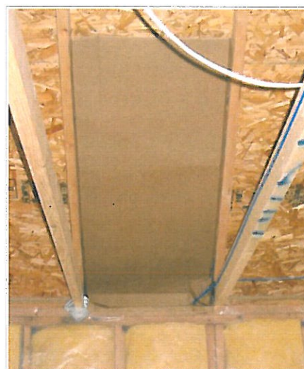
R402.2.3 Eave Baffle Baffle at eave vent. Minimum 1" unobstructed air space required.
