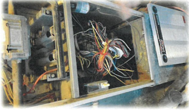
(Furnace in need of replacement)
