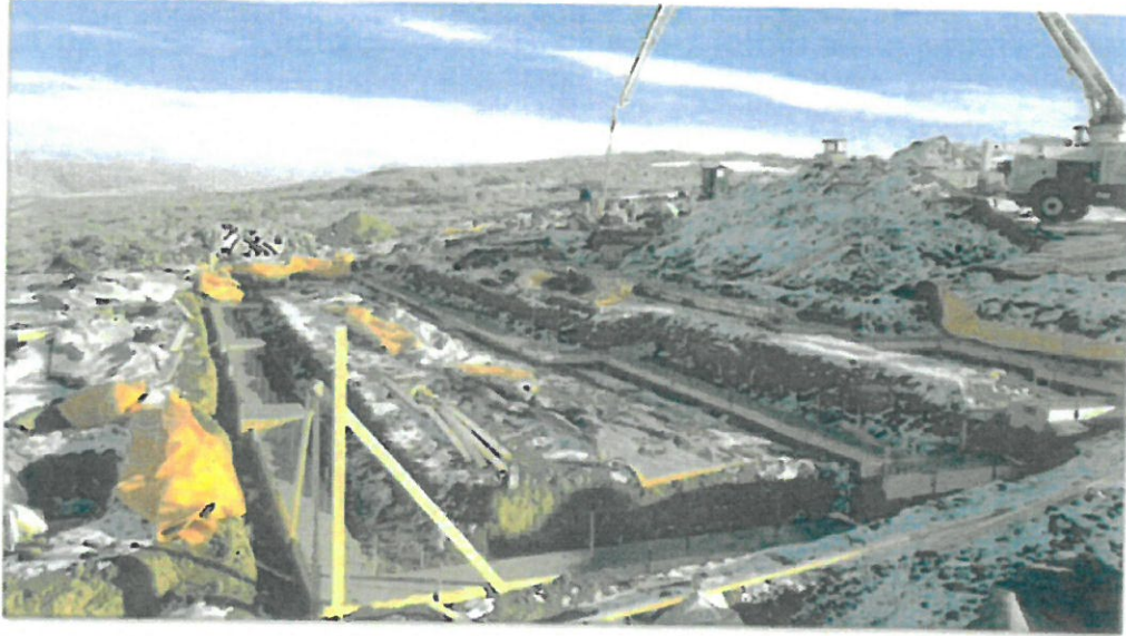
Photo taken by William Longmire of contractor pouring garage footing the same time as house footing on 12/27/2018.
