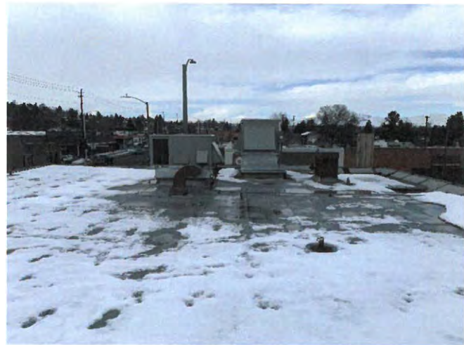
A photograph of the roof upper roof with HVAC units
