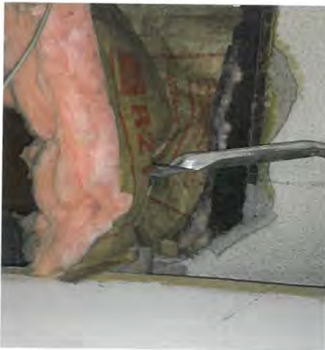
Water damage from roof leak at teller window
