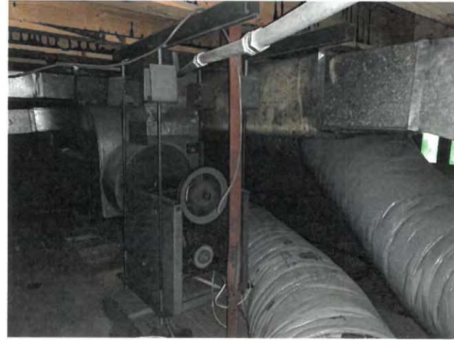
The HVAC system within the attic space.
