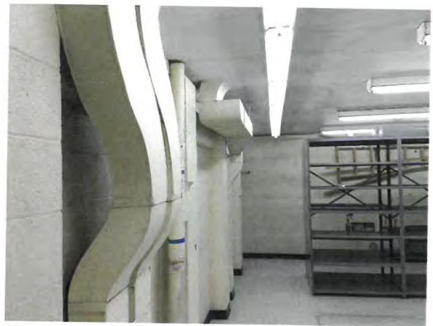
Traces of dust/residue on ceiling in Storage Room
