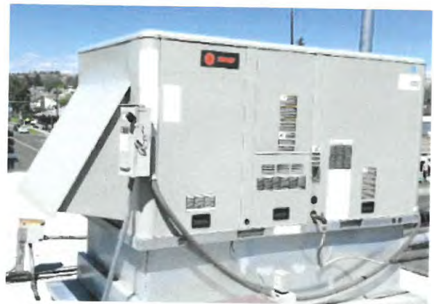
Roof top HVAC unit, gas fired (serves first floor)
