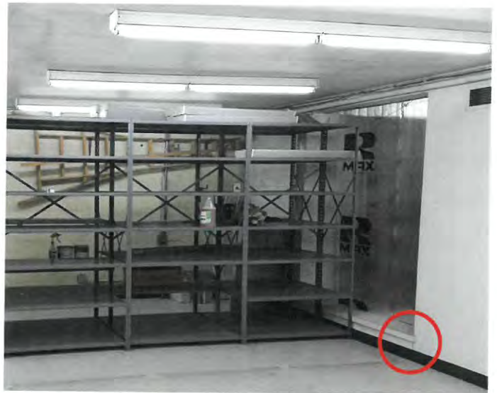
Storage room (location of crack is circled)
