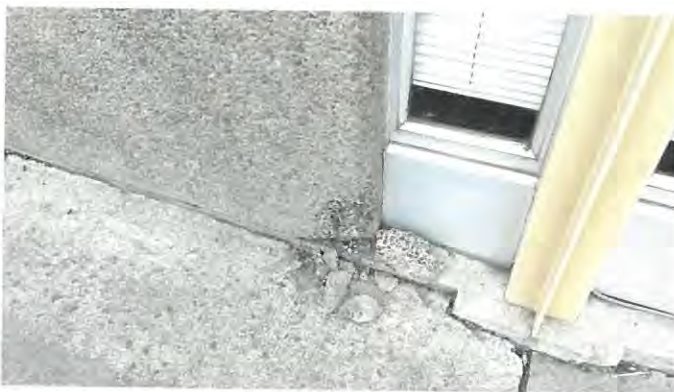
Cracked and spalled corner of precast panel
