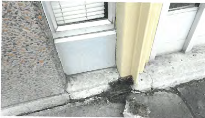
Rust at bottom of steel column and spalled portion of concrete base
