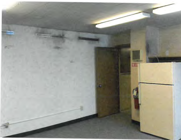
Dust/residue around diffusers (Second floor)
