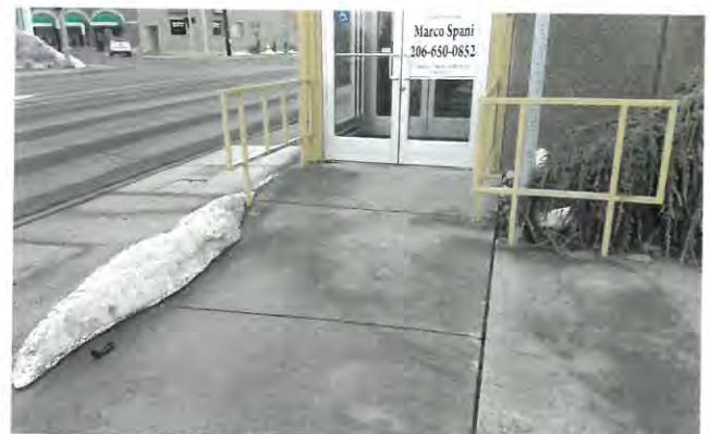
Steep slope at south entry
