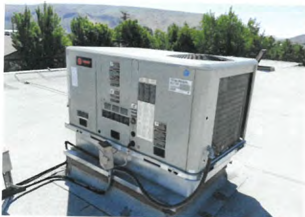
Roof top HVAC unit, gas fired (serves second floor)
