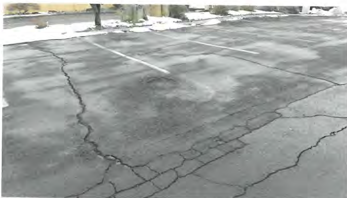
Alligator cracking in parking lot
