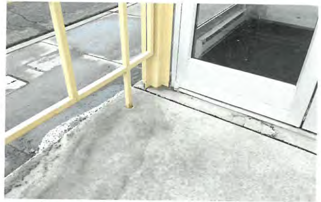
Rust at bottom of steel column and handrail post
