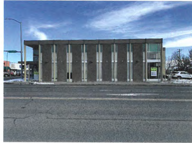
A photograph of the west exterior side of the building. The windows contain ACM window putty and glazing.
